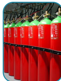
Fire Fighting System
